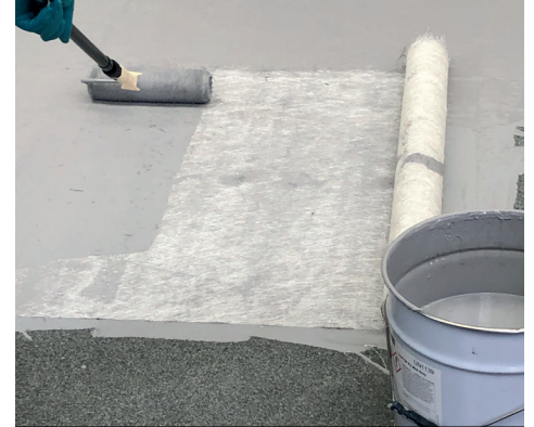
The field area of the roof then receives the embedment coat and reinforcement.
