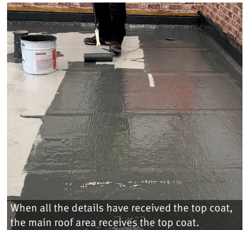
The pipe penetration receives the PU top coat and the weather edge adequately protected.
