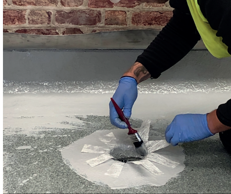
Embedment coat and glass fibre mat are dressed into the throat of the existing outlets.
