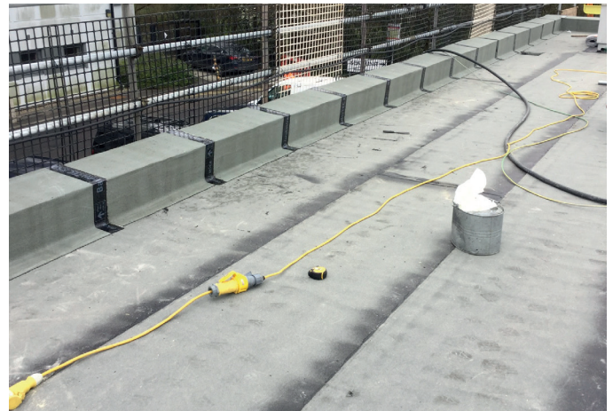
AVCL taken to full extent of upstand
