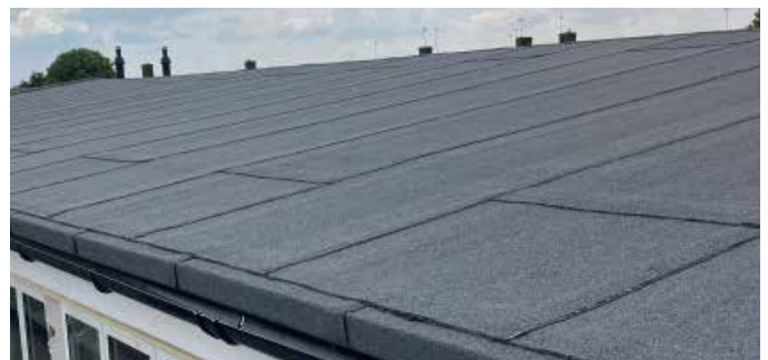
Image of welthed drip to external gutter
