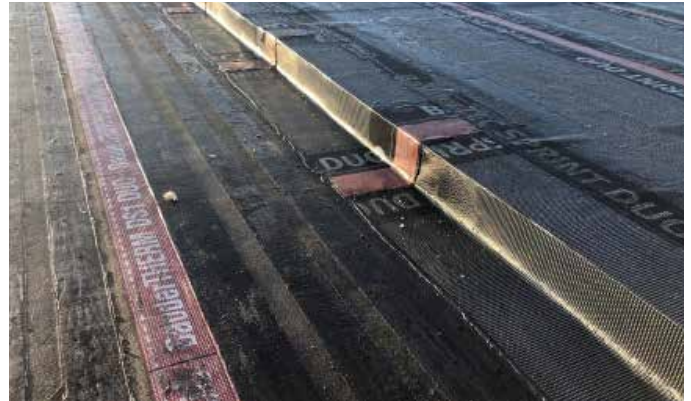
DS 1 DUO installed to field area
